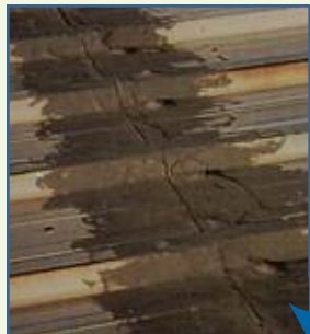
Fix seam and fastener problems
